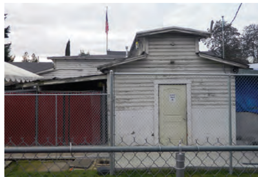
Rotting eaves will be replaced to stabilize the structures
